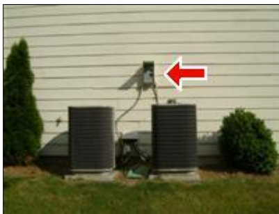
11.11 Picture 1 A/c disconnect
