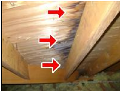
1.0 Picture 1 water stains
