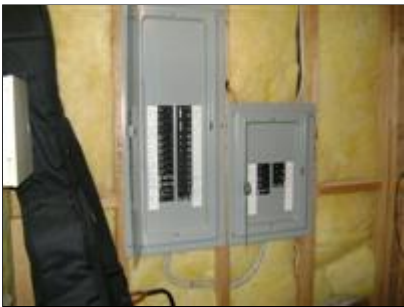
9.1 Picture 1 Main and sub panel
