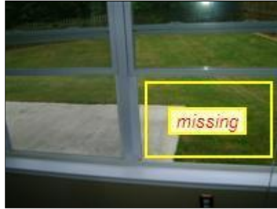
4.6 Picture 1 Screen missing
