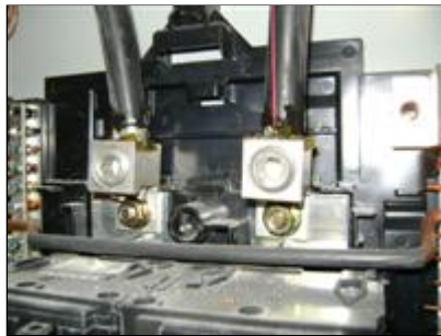
9.1 Picture 2 Service conductors
